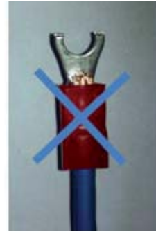
Terminal has been cut.
